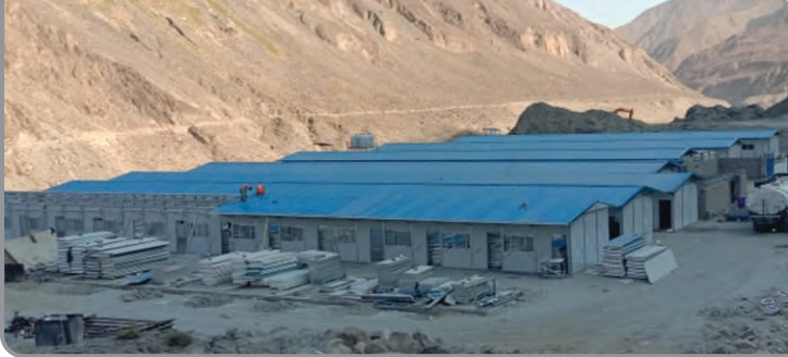
Power China | Temporary Accommodations 38,000 Sft
