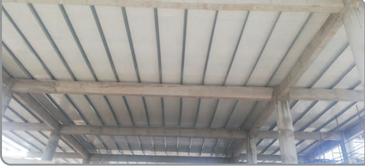
Rajby International | Roof Panel System 28,000 Sft
